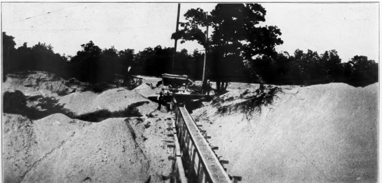
View of Conveyor Passing Under the Road to the Hopper in the Background
